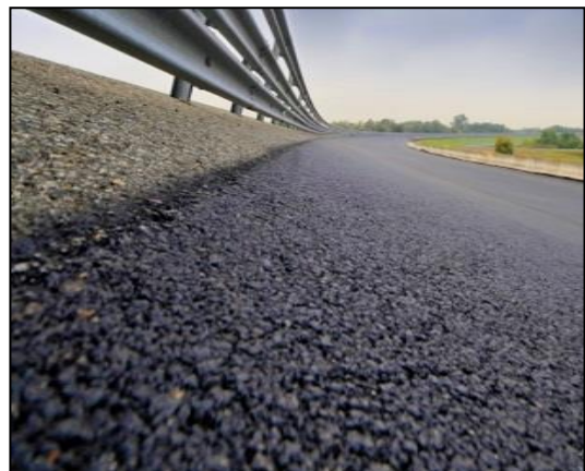
Figure 5: Segregation due to defective
