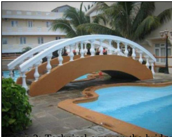
Figure 2: Technical error on the bridge. balcony.
